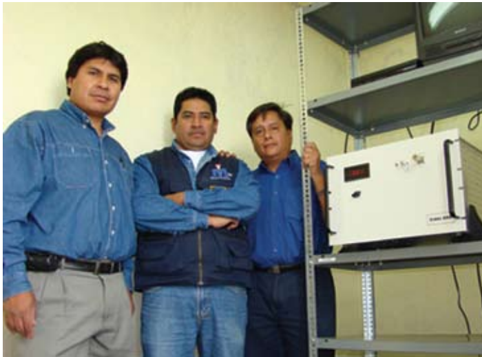
Headend Technicians Jesús Vedia and Ángel Sánchez with Engineer Juan Carlos Baya following installation of the Repeater
