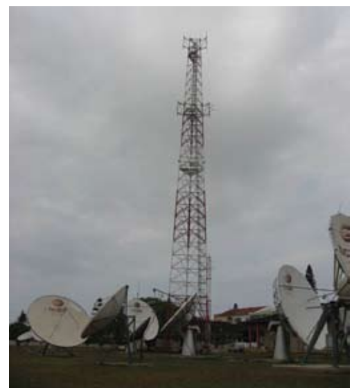
Base Station antenna in Maputo, the capital city of Mozambique.
