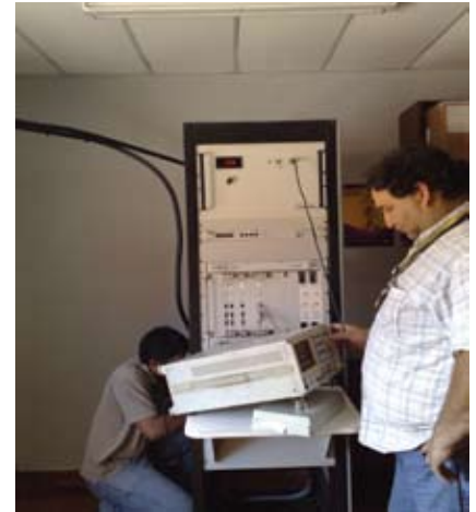
Carlos Esteche and Miguel Orsua testing the fiber optic and base station transceiver equipment.
