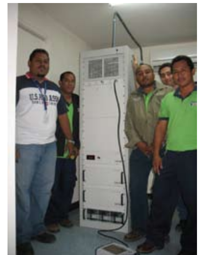
Iran Tejada (left) with the technical crew from Cable Onda following commissioning of the 1000 Watt transmitter
