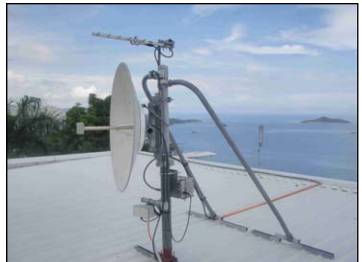
Upstream Bi-directional Repeater Installation at one of Hitron's repeater sites
