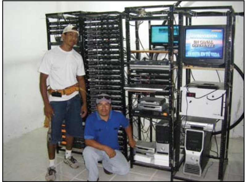
Technicians from Cable Zar finish installation of the MMDS transmitter in Galapagos, Ecuador
