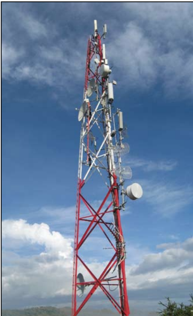
Antenna tower at Port Moresby, Papua New Guinea
