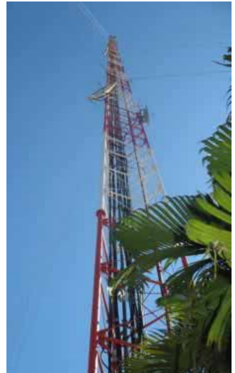
Repeater antennas mounted on the repeater tower.
