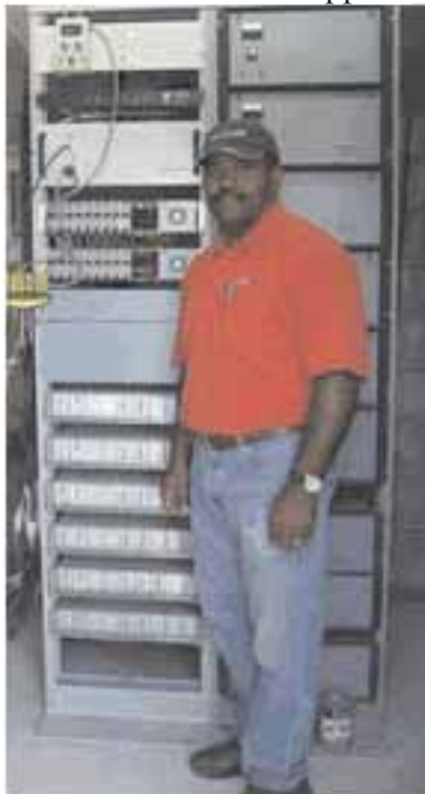
Elvis Brown of Cable One installs the headend hardware for the Multichannel HDTV Link.
