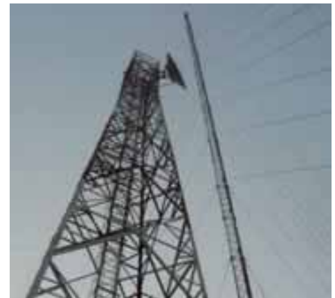
Relay station towers at Sahiwal are 55 Kms from Main Transmitter at Renala Headend.
