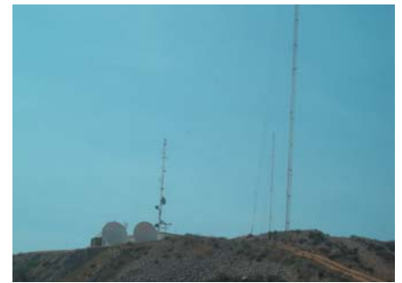
Cerro Jaramillo headend installations showing satellite receive antennas and STL antenna
