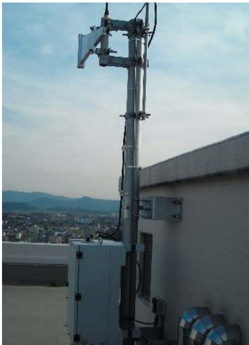
“Triple Play” Base Station Transceiver and Sector Antenna.
