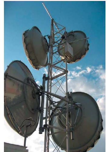
13 and 18 Ghz Antennas at Guthrie Peak repeater site
