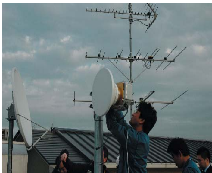
Takashi Eifuku from V-Network Systems adjusts one of the remote subscriber antennas.
