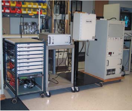
Digital Headend, STL, and MMDS System Test
