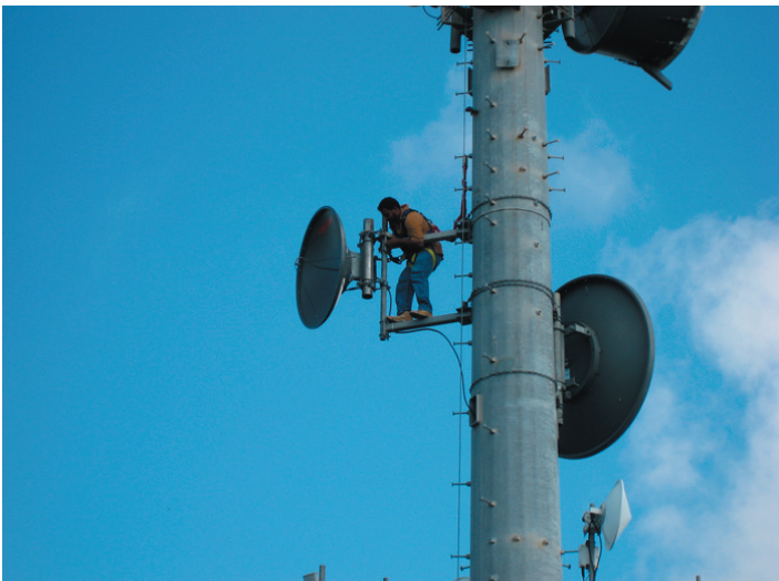
Anthony Ramirez adjusts the 4 foot 18 GHz receive antenna at the St. Georges repeater site.
