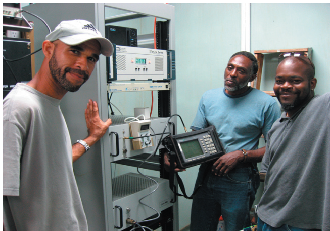
From left to right, Bernard Rey, System Engineer of Innovative Cable in St. Thomas, Douglas Pompey, System Engineer of Innovative Cable in St. Croix and Toya Malone, Media Director for the Government of the USVI, at the Inter-island 13Ghz QPSK transceiver in St. Thomas.
