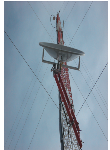
New tower in Fresnillo, with the 13 GHz STL antenna and the MMDS antennas.
