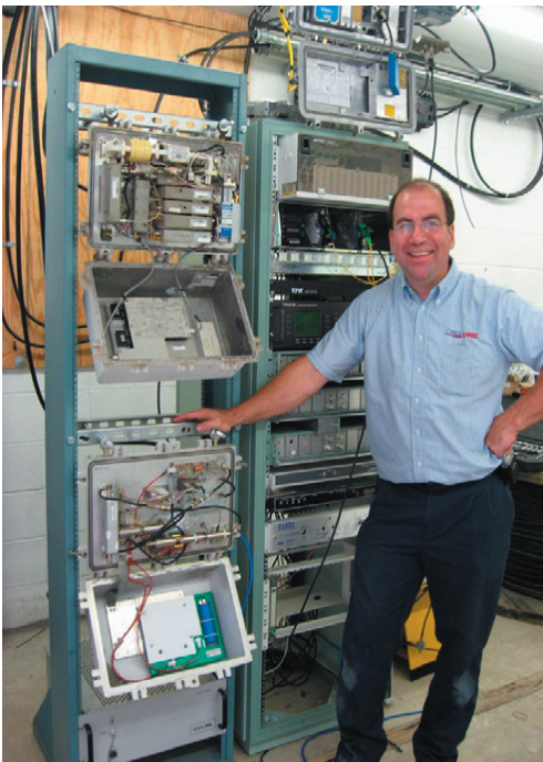
Kenny Wright, System Engineer for Cable One of Natchez MS, at the Vidalia site in Louisiana. Continued on page 4
