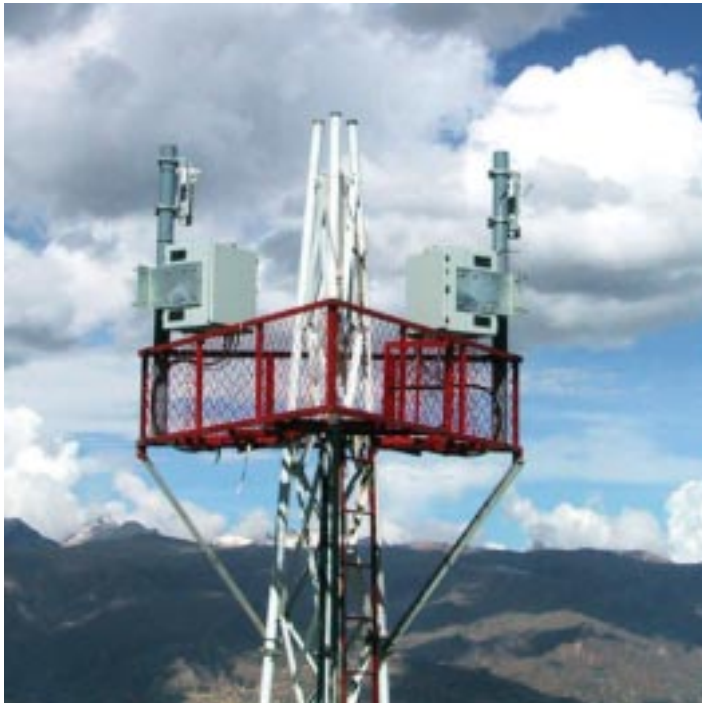
28 GHz Tower Platform Base Station with Outdoor High Power Transceivers and Sector Antennas
