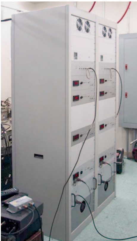
Upgraded Cable AML Broadband Transmitters
