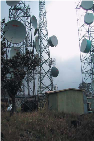
Microwave Antennas from Maui Headend.
