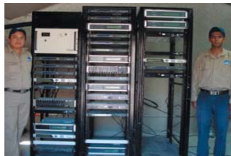
Erick Rodriguez and Jose Hernandez of TV ZAC following the installation of the MMDS transmitter and the Rio Grande Headend.
