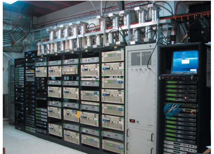
Univisa Headend in Guayaquil showing new broadband digital MMDS transmitter (center) right next to older channelized analog transmitter array.
