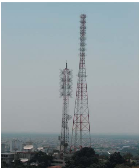
Univisa MMDS transmitter tower in Guayaquil, Ecuador
