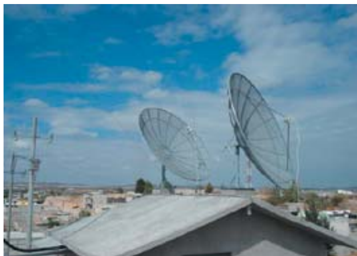
View of the city Rio Grande from the roof of the new MMDS Headend building.
