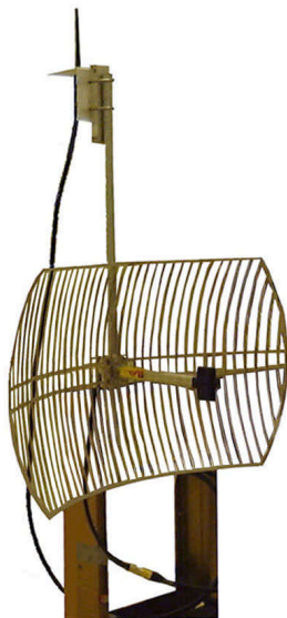
Upstream site of 2.4 GHz FM Mini-Link set up for performance testing
