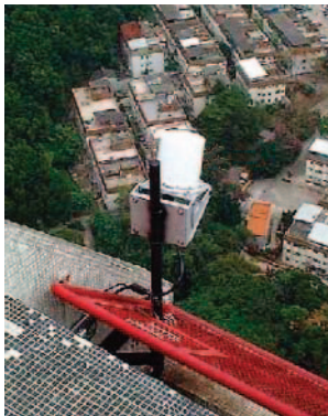
18 GHz Repeater with Sector Output Antenna.
