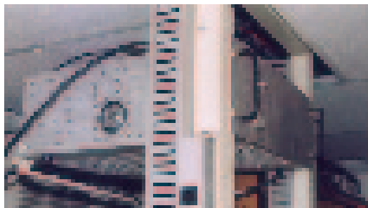
AML ITX-015 transmitter in continuous operation since 1993.
