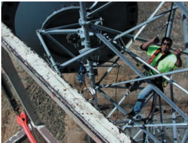
Comcast personnel align one of the antennas in the Rio Vista system.
