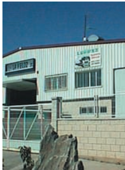
Remote antenna mounted on roof of Industrial Park building.
