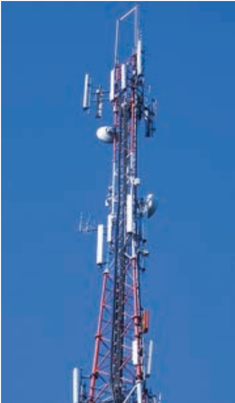
Main tower with STL remote antennas and 28 GHz Transceivers.
