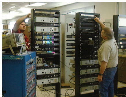
Integrated headend is tested by Cable AML engineers prior to shipping.
