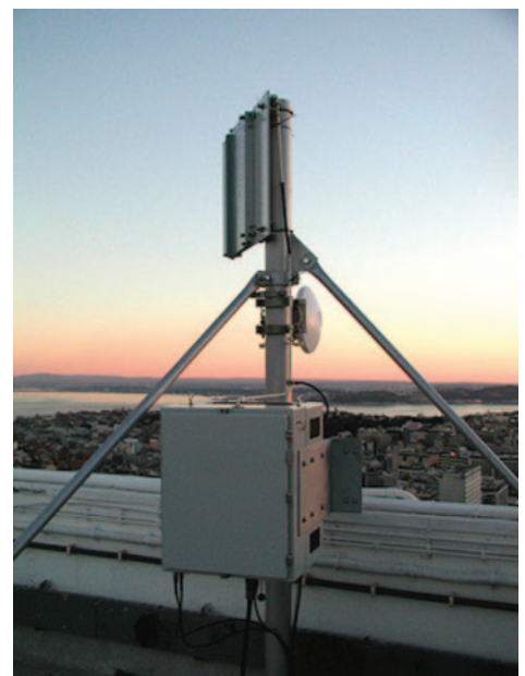
Multimedia 28 GHz Base Station Transceiver installed in Lisbon (Portugal)
