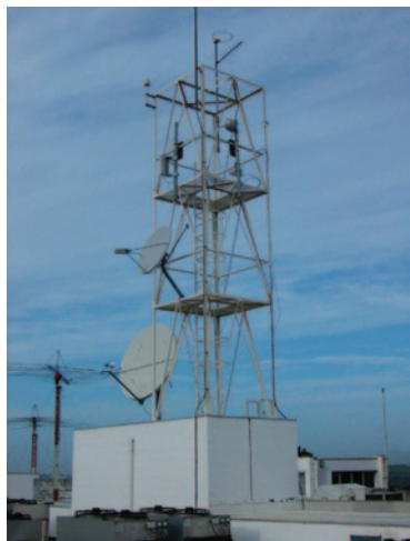
Two-way 28 GHz repeater mounted on top of existing tower for satellite receivers.
