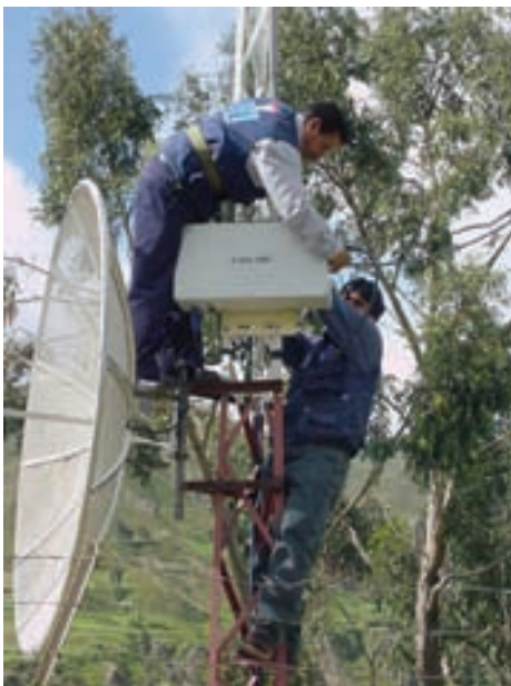
Nicolas Bautista (left) and Richard Tambo (right), of Multivision S.A. install a broadband high power repeater in Chijipata (La Paz, Bolivia).
