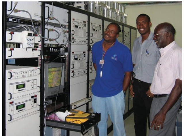
CBC engineers Jeffrey Chandler, Maurice Bailey, and Hallam Franklin checking out the equipment after installation.
