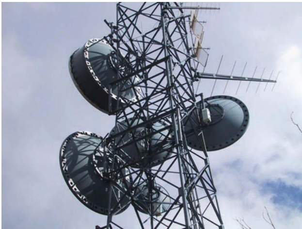
Repeater tower at Mingus Mountain
