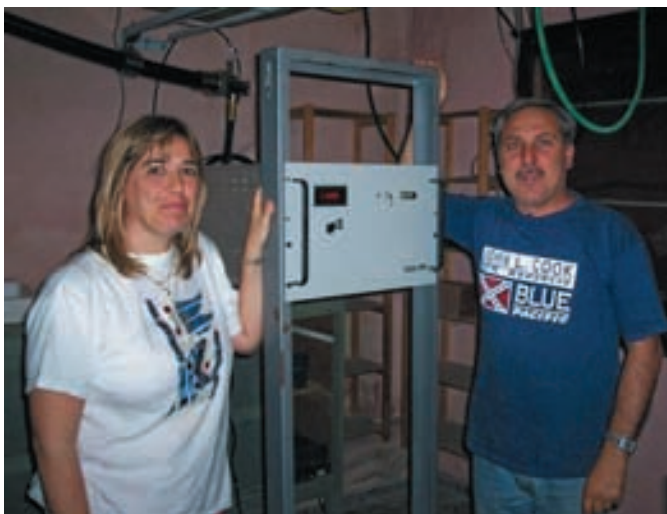
Laura and Ramiro Lobecio during commissioning of Cable AML transmitter.
