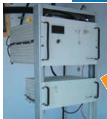
Repeater site 30 Kms from San Luis Colorado houses an Indoor Repeater fed by a Point-to-Point MMDS link from the main transmitter.
